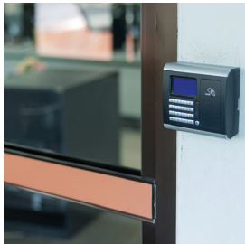
Access Control System
